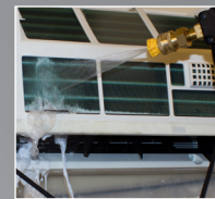
Clean coils from the front
