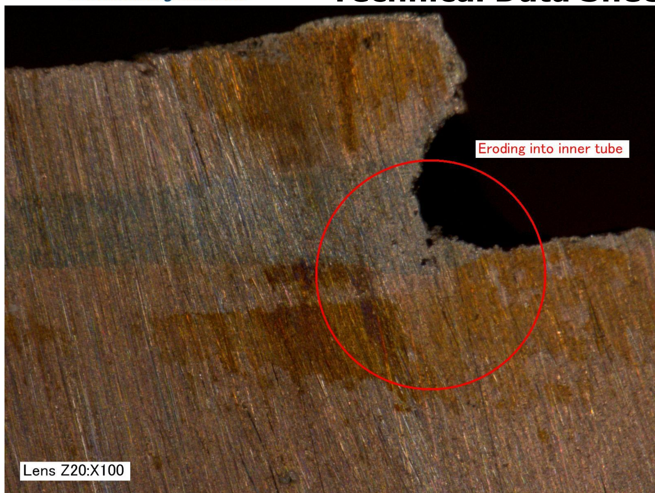
Figure 1: Erosion of Sil-Fos into Copper base metal
